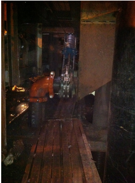
Figure 2 – Slurry volumetric flow rate measurement tank.
